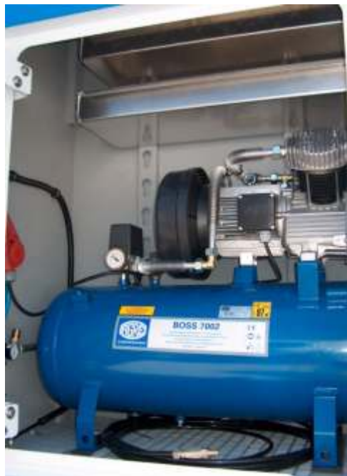
Compressor for the usage of diverse pneumatic machines/ devices
